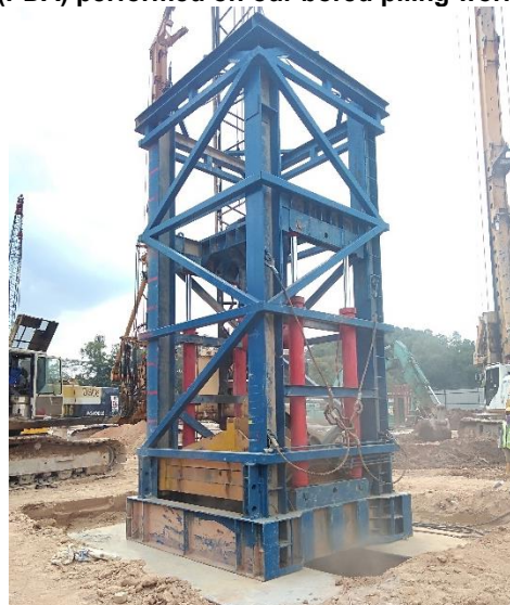
Dynamic load test using the Pile Driver Analyzer (PDA) performed on our bored piling works
