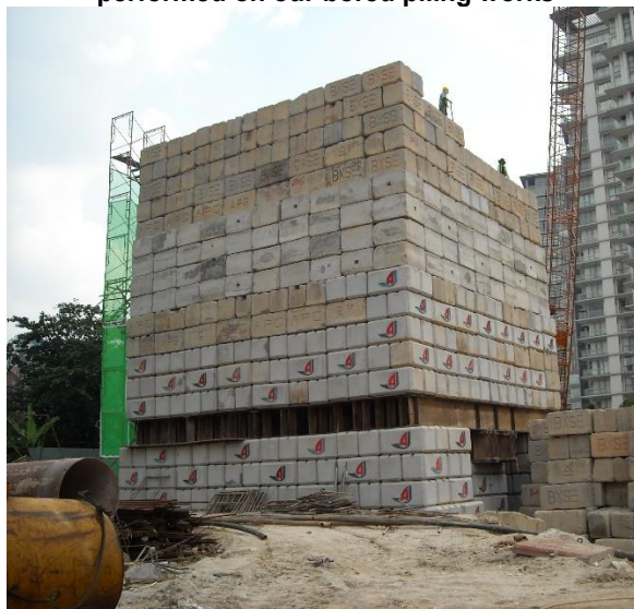
Static load test using the Kentledge system performed on our bored piling works
